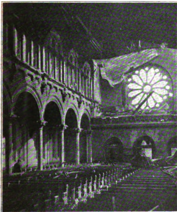
VIEW TOWARD THE REAR. ROSE WINDOW, BROKEN, IN THE DISTANCE. ONLY ONE WINDOW ON NORTH SIDE IS DAMAGED
