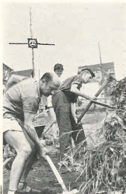
TRAINED WORKMEN joined young people on some projects and at one German camp invited them home for tea and meals. Cut shows terracing of grounds around a church and playground at a Saar Work Camp. Cross in left background bears seal of the World Council.*
