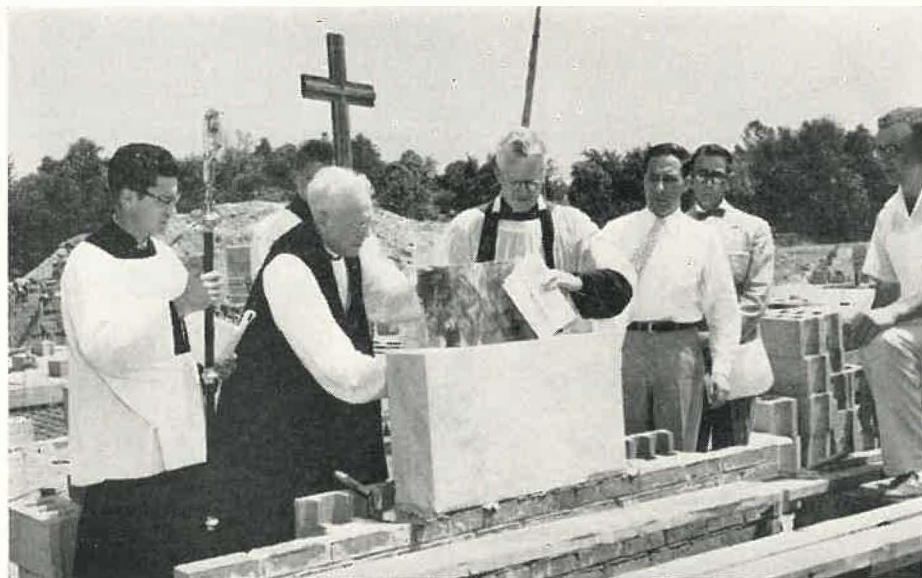
PLACING OF THE SEALED copper box in cornerstone laying ceremonies at St. Michael and All Angels Church, are (from left): Charles Culley, bishop's chaplain; Ron Freeman; Bishop Kirchhoffer; the Rev. George Evens, rector; Charles Saletta, architect; Henry Rohmann, building chairman; Guthrie Whistle.
