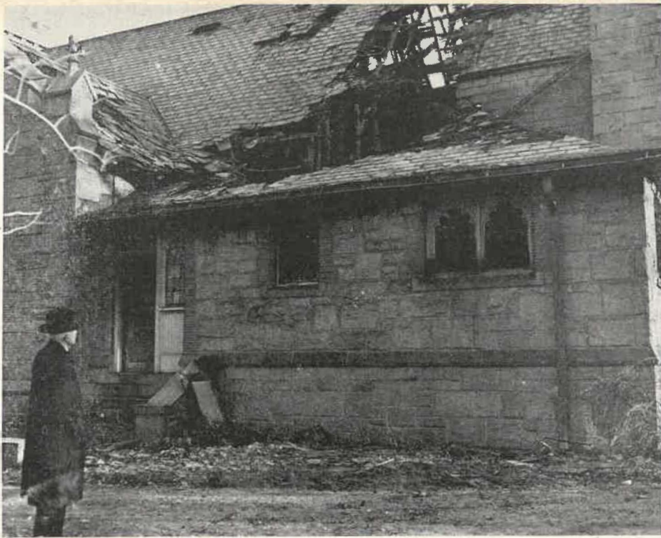
Rev. Fred Sutton, rector, checks exterior damage caused by fire to Church of the Good Shepherd.
