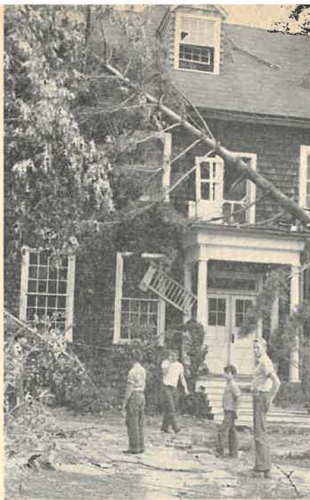
Students of the Church's Blue Ridge School, St. George, Greene County, Va., looked over the destruction performed by a tornado which damaged almost every structure on the grounds, September 30th. This is Mayo Hall, which houses classrooms and administrative offices. Forty children barely escaped injury in the storm [L.C., October 11th]. School officials estimate repairs will cost $100,000 to $250,000.
