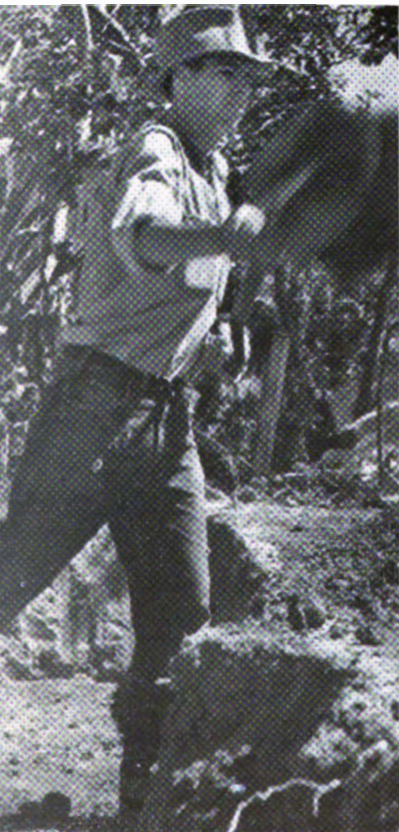
A work camp member in Mexico begins work for a foundation of a brick building in one of the villages.
