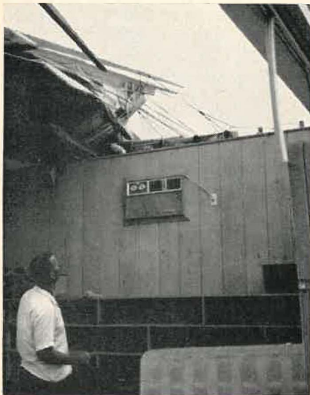
Fr. Cox and storm damage Water at their feet; water from the ceiling.
