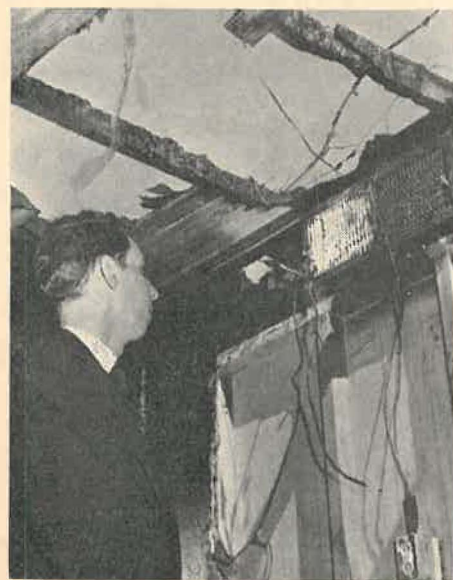
A fire-blackened ventilator and a hole in the roof indicate the plight of St. Mary's Church, Phoenix, Ariz., which was badly burned last month [L.C., April 28th]. The Rev. Lewis H. Long, rector, is shown inspecting some of the damage. Cause of the fire has not been determined.
