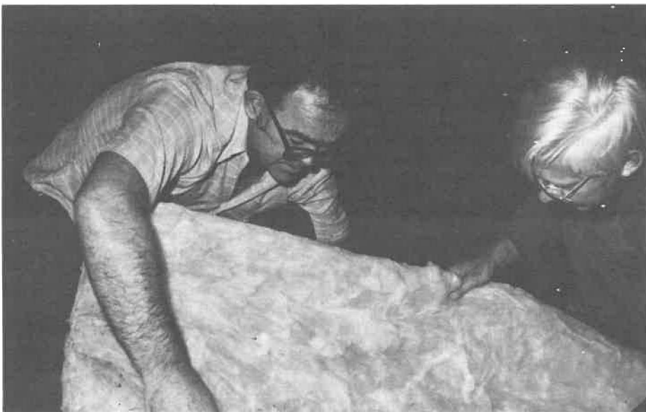
Mr. Gene Rizzo (left) and Mr. James Lewis add insulation to the church structure.
