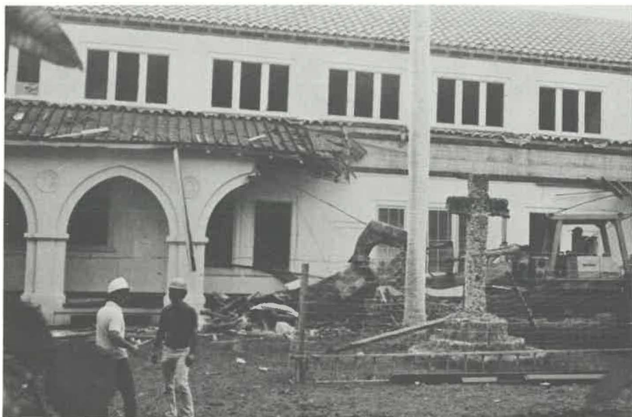
The beginning of renovation of Kennedy Hall at St. Andrew's Priory School, Honolulu, Hawaii.
