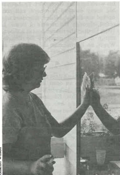
Sherri Simon cleans a newly installed storm window on a house in Brown County, Ohio, at the APSO/Youth's workcamp.
