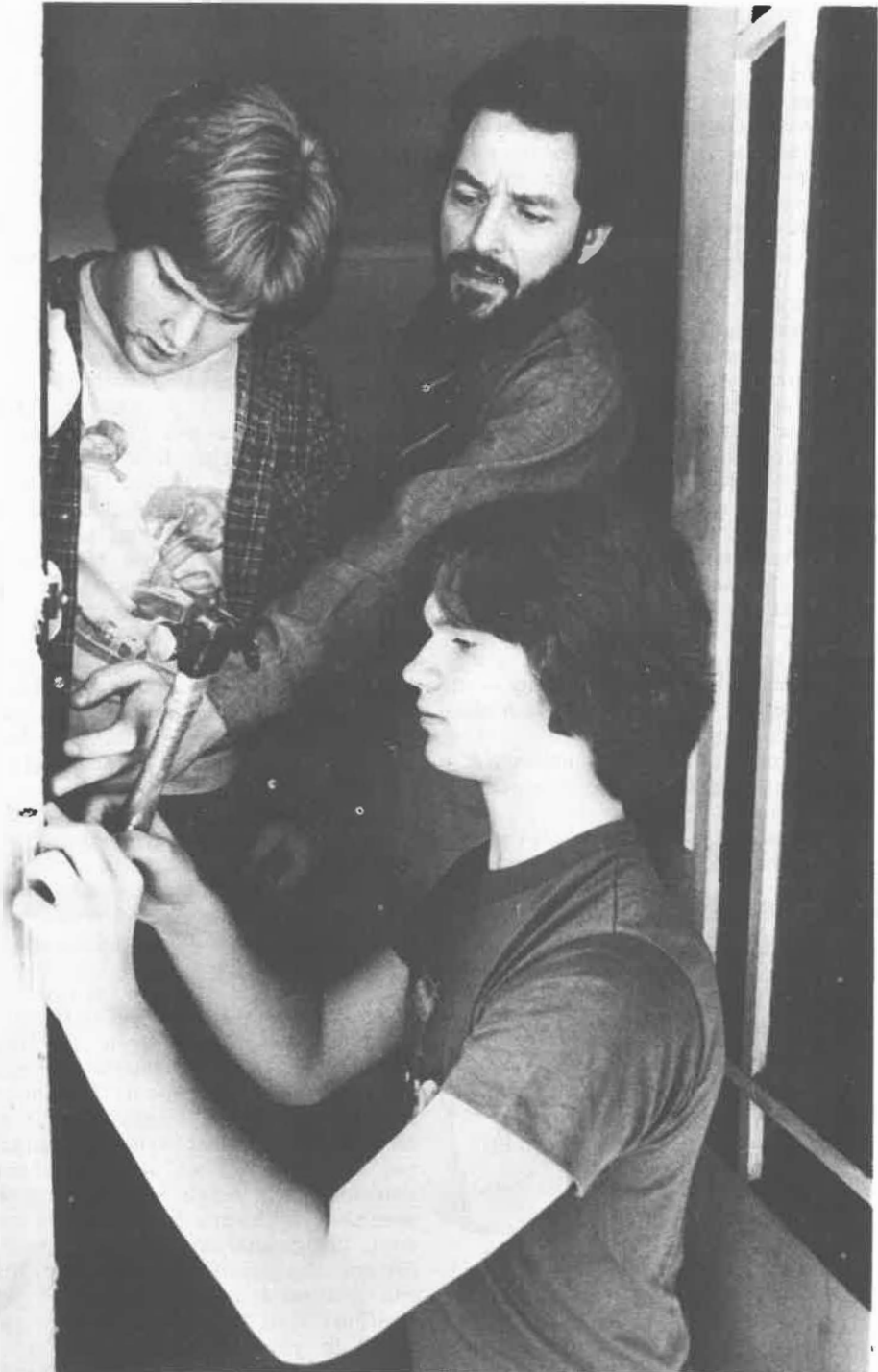
Volunteers John Tanner, Bart Stokes, and Scott Hutchinson of the Church of St. James the Less, Nashville, nail weatherstripping to the door of a home whose owner is not able to do the work himself [see p. 6].
