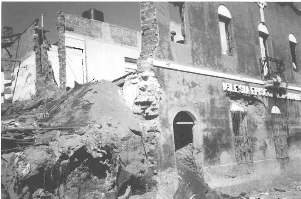
An Episcopal church damaged by Hurricane Mitch.
