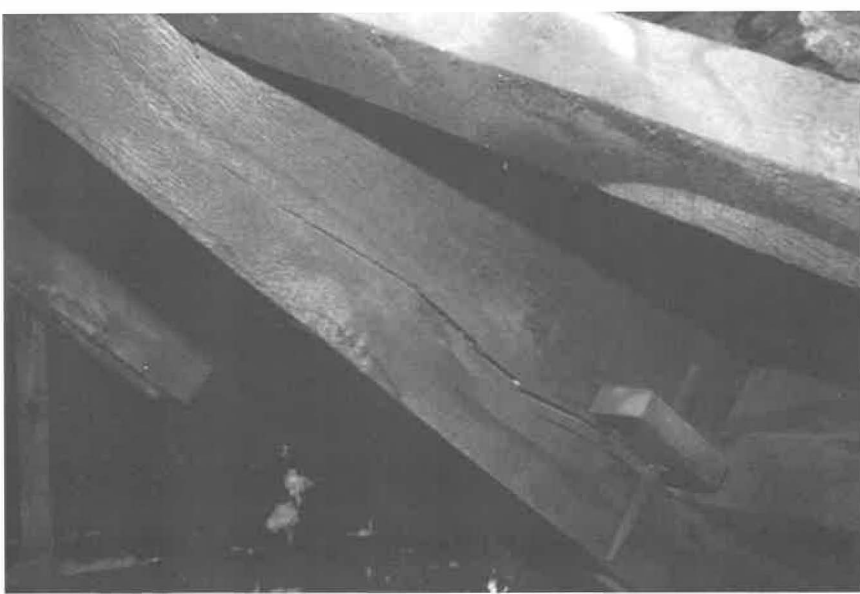
Counter-clockwise from top: Trinity (Old Swedes) Church, present; crack in truss; repairing the roof; carpenter fitting new steeple rafters; engineering inspection of basement.
