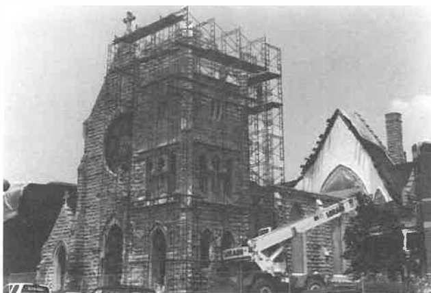
Trinity Church, Clarksville, Tenn., is being restored after it was heavily damaged by a tornado in January.
