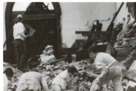
Parishioners sort through the rubble of a church damaged by a tornado. Metaphor for our times?
